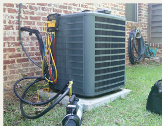
Pre-season HVAC tune ups
